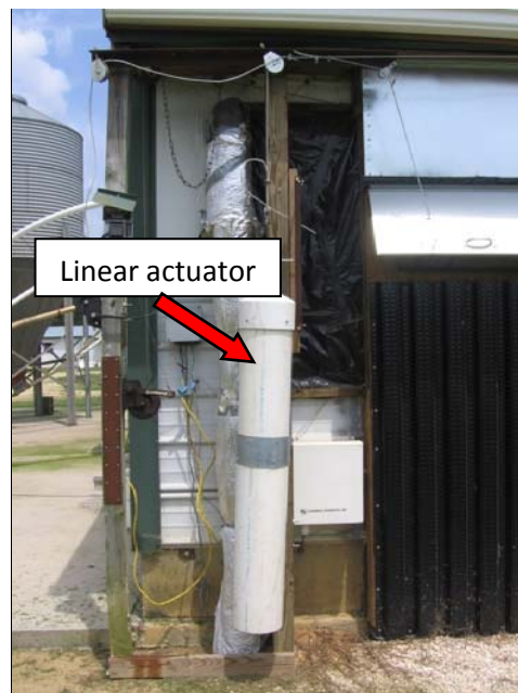
Figure 2. Picture of the linear actuator used to operate the dampers to bypass the TSW
