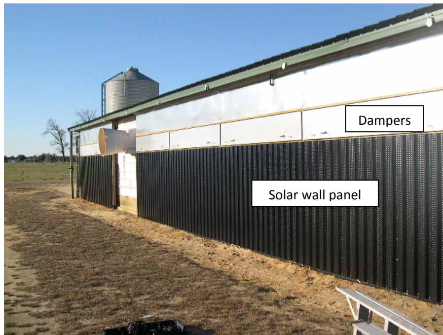
Figure 1. Solar wall installed on the south side of a pig nursery on the N&J Butler Farm near Clinton, NC
